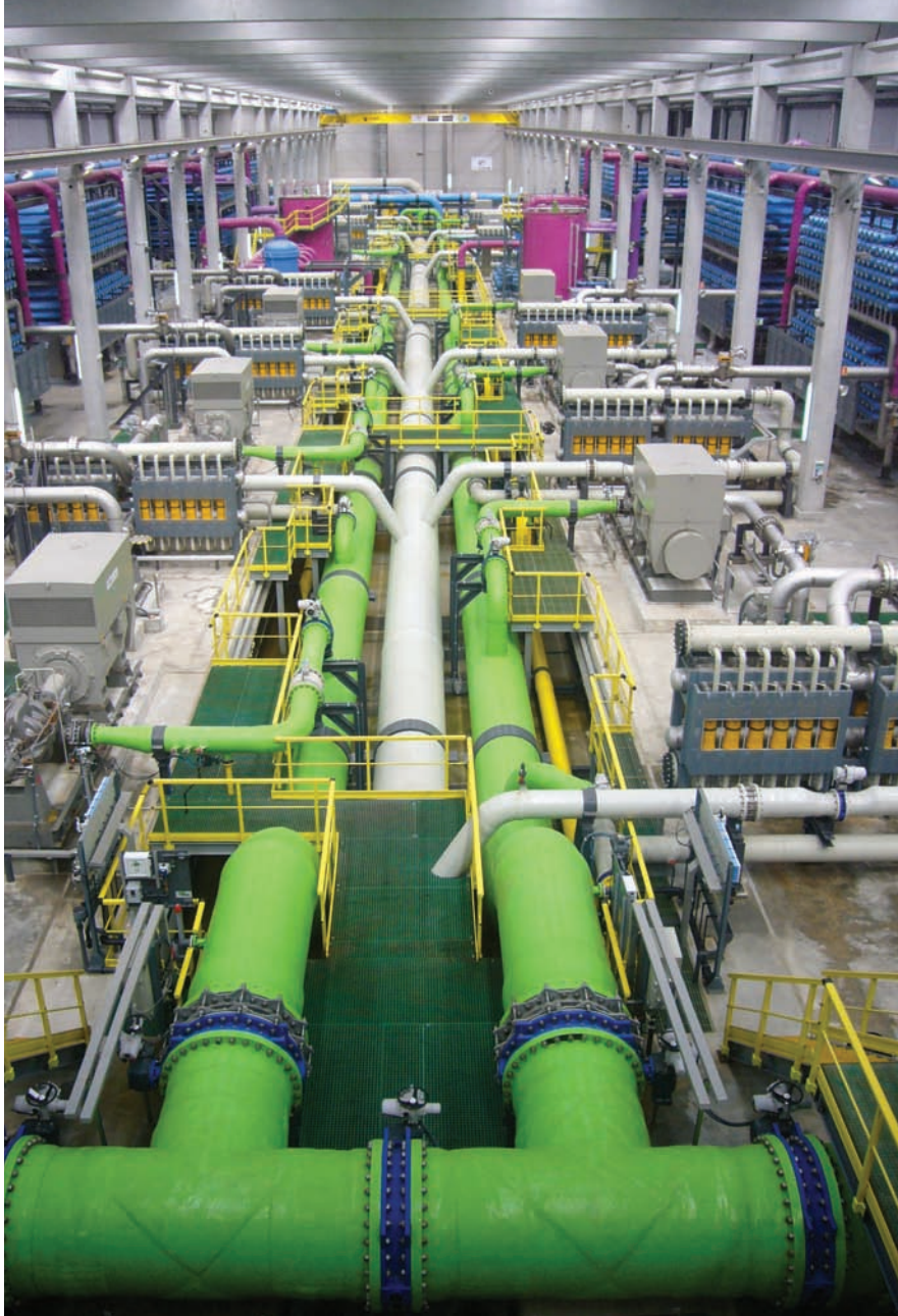
A reverse osmosis desalination plant in Barcelona, Spain.
