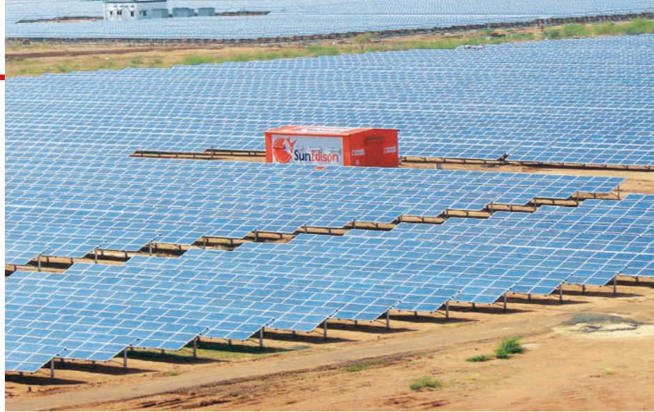
Charanka Solar Park in Gujarat has equipment from the US and China
